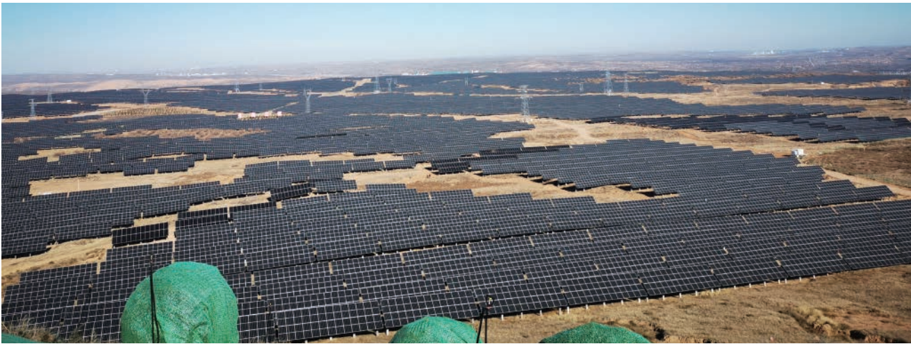
Inner Mongolia, China Completed: 2021
